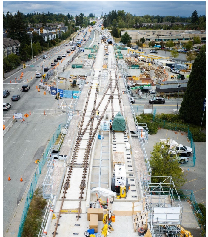
Aerial view of switch section located at 166 Street.
