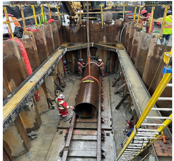
Figure 4: Crews installing an underground duct bank under a rail crossing that will house electrical lines to power the future SkyTrain.
