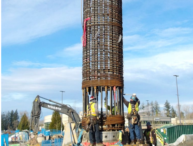
Figure 1: Ongoing foundation construction at the site of the future Bakerview - 166 Street Station.
