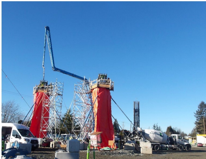
Figure 3: Construction of piers that will support the future elevated guideway at 152 Street Station.
