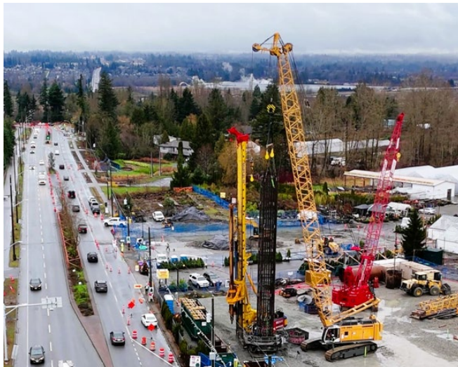
Figure 3: Foundation construction continues at the site of the future Hillcrest-184 Street Station.
