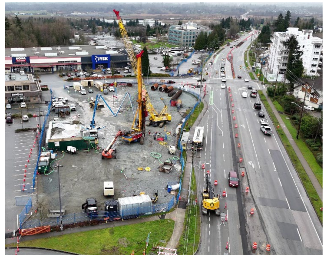
Figure 4: Foundation construction underway at the site of the future Bakerview-166 Street Station.
