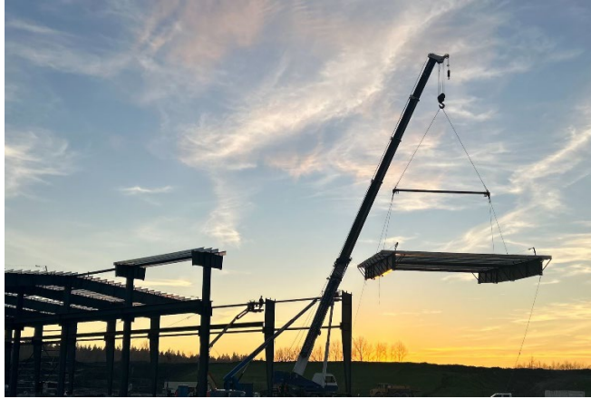
Figure 1: Installation of the columns and roof structure for the production building at the precast concrete facility where the guideway segments will be fabricated and stored.
