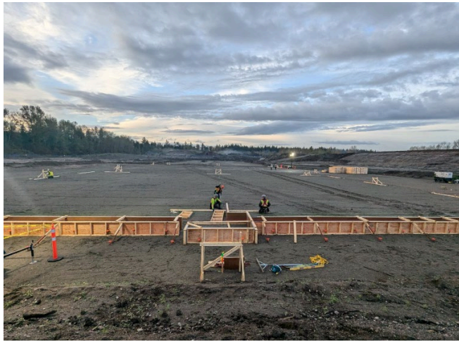
Figure 1 - Site preparation activities underway at the precast yard where Guideway segments will be prepared and stored.
