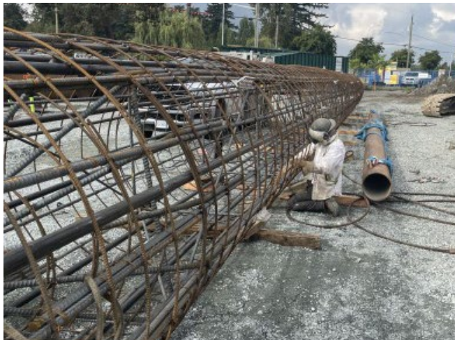
Figure 3 - A rebar cage being built at 184 Street and Fraser Highway to support geotechnical investigations and test piling activities.
