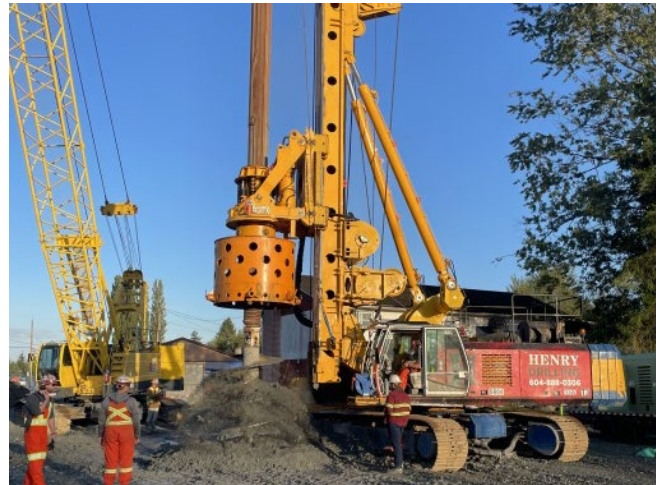
Figure 2 - Test piling activities underway at the Hillcrest-184 Street Station location as part of the geotechnical investigative works.
