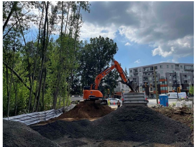
Figure 4 - Vegetation clearing and grubbing underway at the Green Timbers SkyTrain Station location to accommodate SkyTrain infrastructure.
