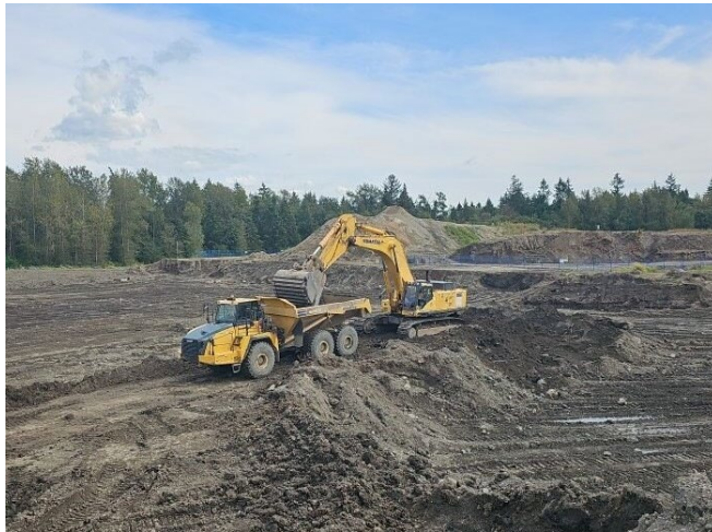
Figure 3 - Site preparation activities underway at the precast yard where Guideway segments will be prepared and stored.
