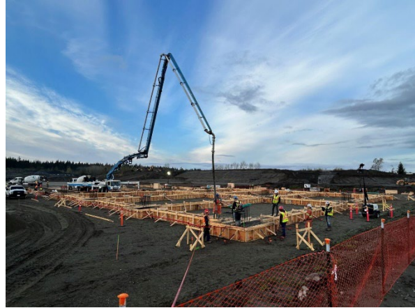
Figure 2: Concrete pour underway for the foundation works of the production building at the precast yard.
