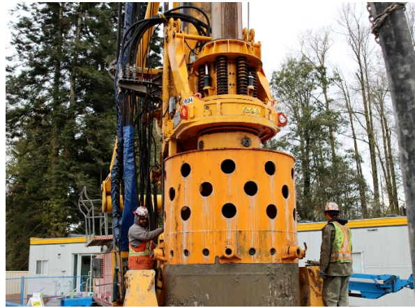
Figure 4: Test piling underway at Fraser Highway and 184 Street to support the future SkyTrain guideway columns.
