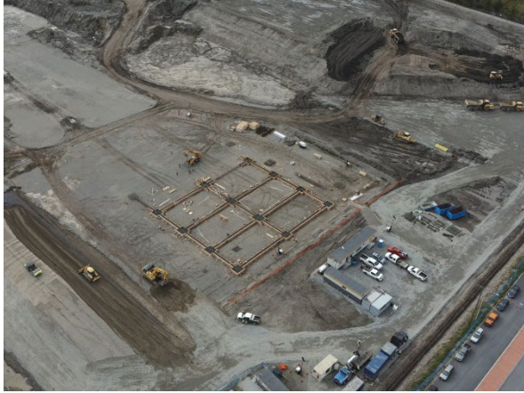
Figure 1: Aerial view of the precast yard preparation where the guideway segments will be fabricated and stored.
