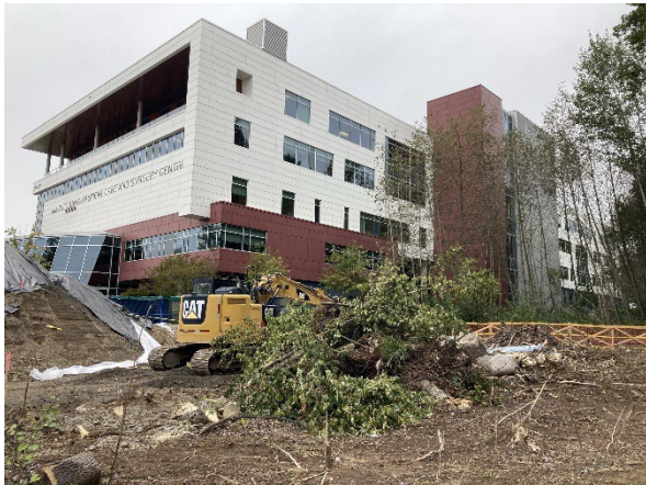
Figure 3: Vegetation removal underway to prepare the site of the future Green Timbers SkyTrain Station at Fraser Highway and 140 Street.
