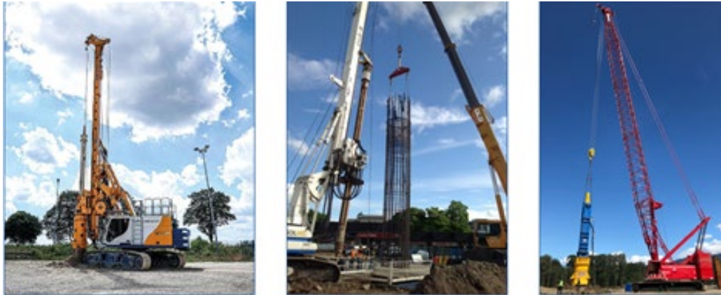
Fig: Mobile cranes and drill rigs will be used for foundation installation.
