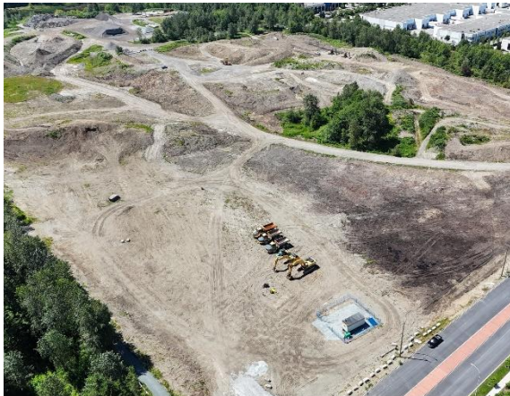
Figure 3: Aerial view of the precast yard preparation where the guideway segments will be fabricated and stored.
