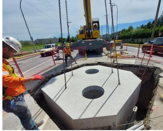
Figure 2: Installation of a four-way vault underway, as part of the BC Hydro distribution line relocation underground works.
