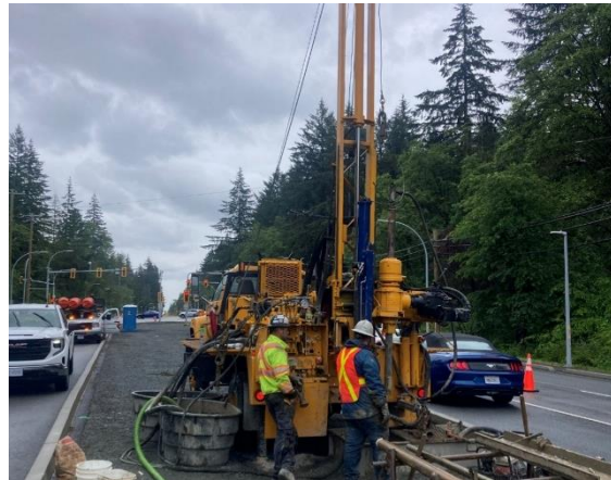
Figure 4: Borehole drilling operations in the median underway on Fraser Highway east of the Green Timbers SkyTrain Station.
