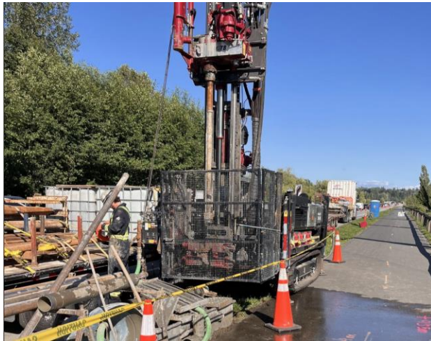
Figure 1 - Borehole investigative works ongoing near the Serpentine River area on Fraser Highway.
