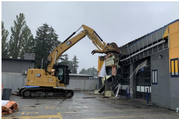
Figure 2 - Building being demolished at 15181 Fraser Highway (former Mr. Lube) to accommodate SkyTrain infrastructure.
